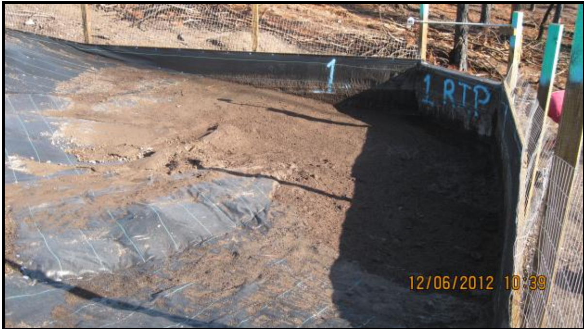
Figure 33. Sediment deposition in fence #1.
