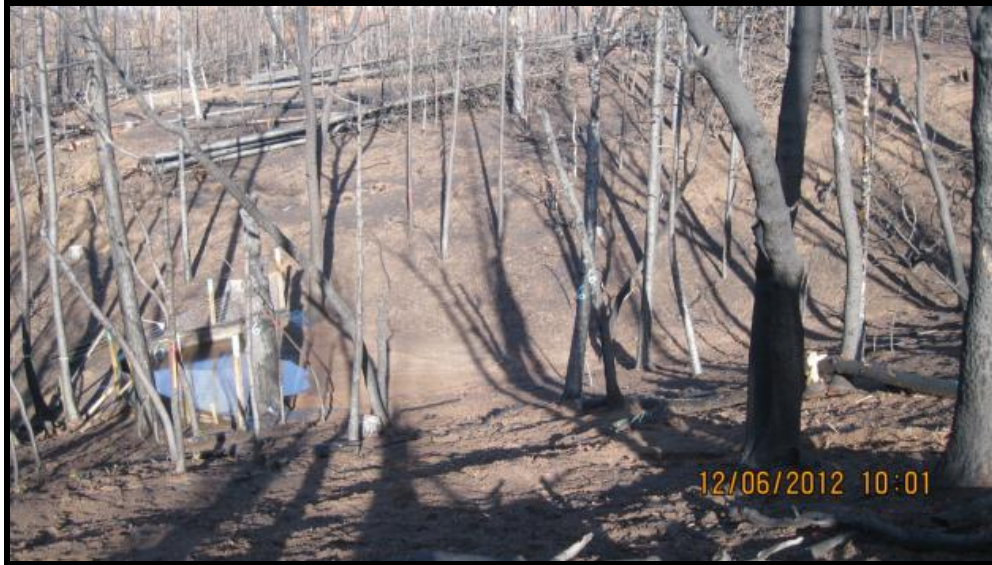
Figure 17. Looking down at fence #6. Note the ponded water in the sediment fence.
