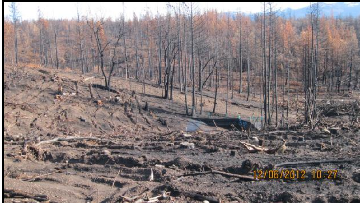
Figure 28. Contour ripping in the lower portion of the swale draining to fence #3.
