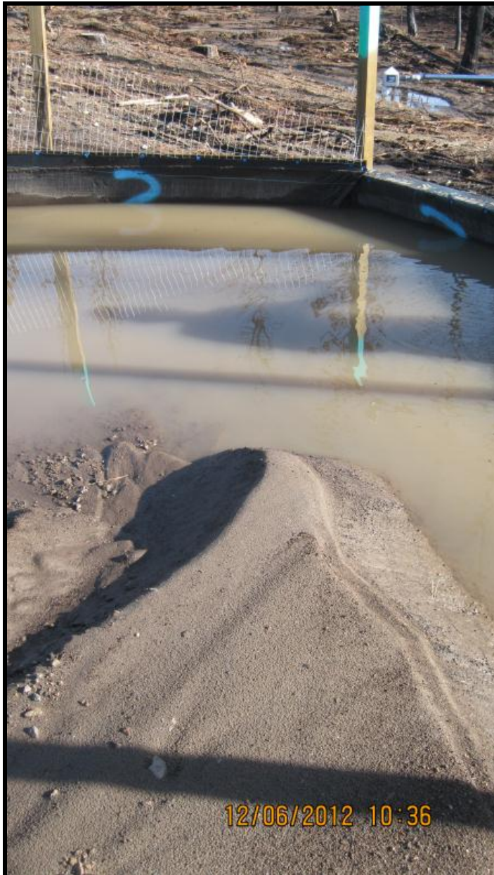
Figure 30. Sediment deposition in fence #2.
